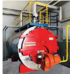
Hot Water Boilers
