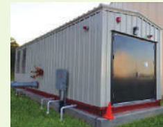
Packaged Fire Systems
